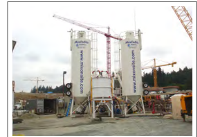
High production equipment
